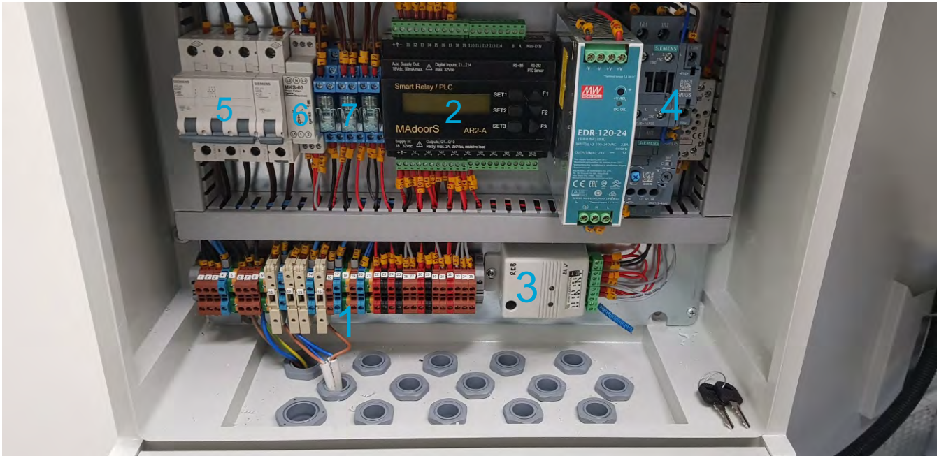
1. Cable connection terminals
